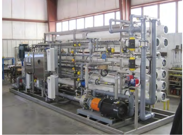
Picture 4.2.5.1: Aqua Innovations Reverse Osmosis System
